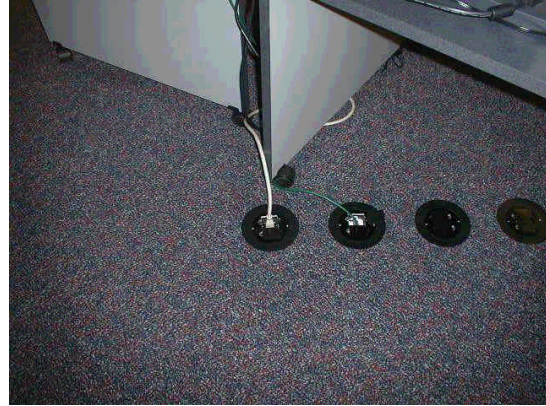
Photo 6: Close-up of the Cat 5 cable exiting the overhead projector and feeding through an opening in the floor to return to the wiring closet.
